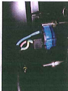
[6] Affected fan - rear of electrical
