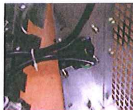
[5] Affected fan - rear of electrical socket & conductors
